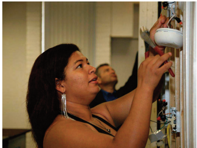
Anais Sevillanos, a graduate of CASA de Maryland’s construction trades training program, participates in an electrical training class.
